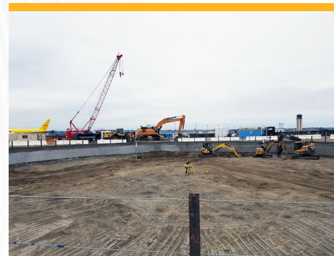
Expanding stormwater system to capture, store and reuse up to 39 million gallons of rain annually.
