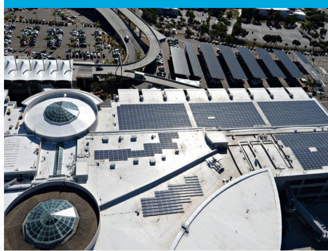
Solar panels on terminal roofs and carports in parking lots generate electric power for the airport.
