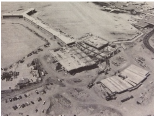
Plate 6.2–2: Construction of Terminal 2 East in 1977. (Courtesy of San Diego Unified Port District 1991)
