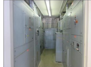
Figure 2-2: Existing T2E Electrical Room
