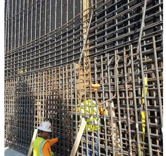
Tons (literally) of steel rebar being placed to allow concrete walls to withstand external pressure without cracking
