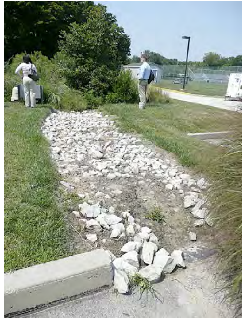
A sediment forebay provides pretreatment for parking lot runoff entering a bioretention cell at Villanova University, PA.
