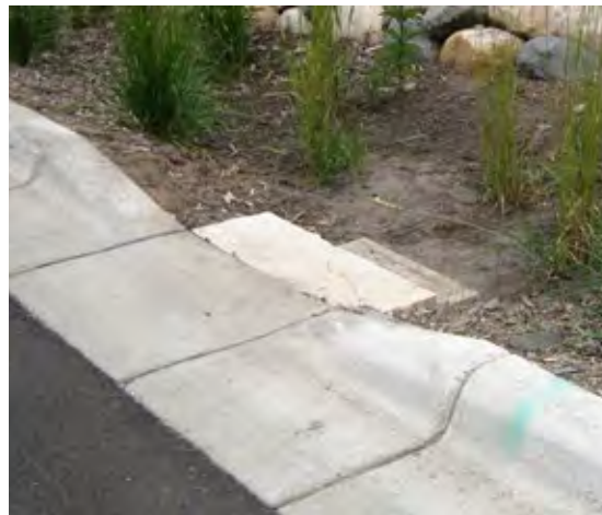
Figure 4-26. A wide-angled curb cut with an energy-dissipating splashpad also serves as access steps for maintenance in Maplewood, MN.
