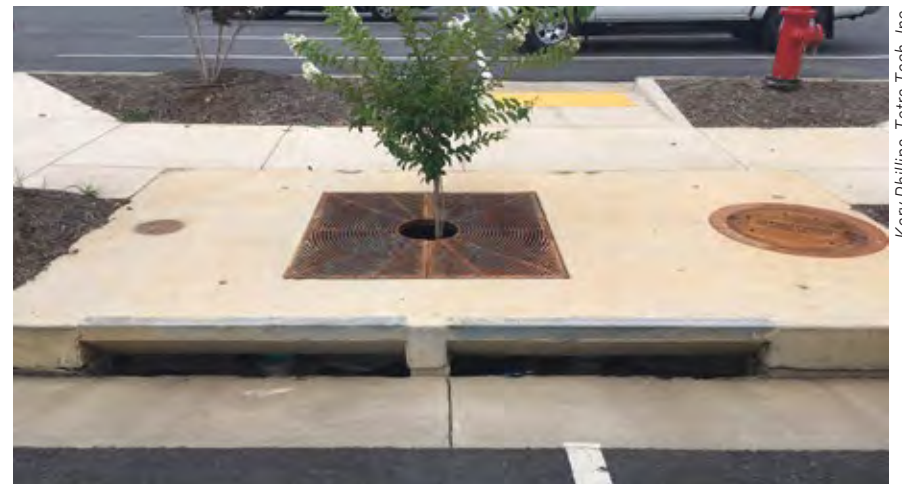
Stormwater catch basin tree pit, Charlottesville, VA.
