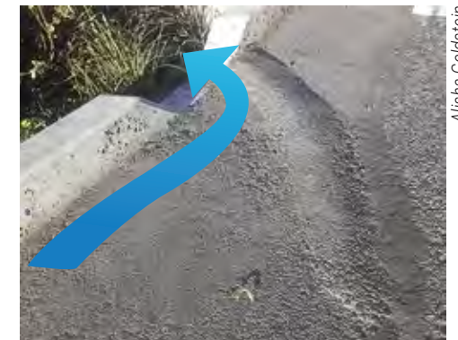
Figure 4-3. A runnel directs stormwater flow, San Juan Island, WA.
