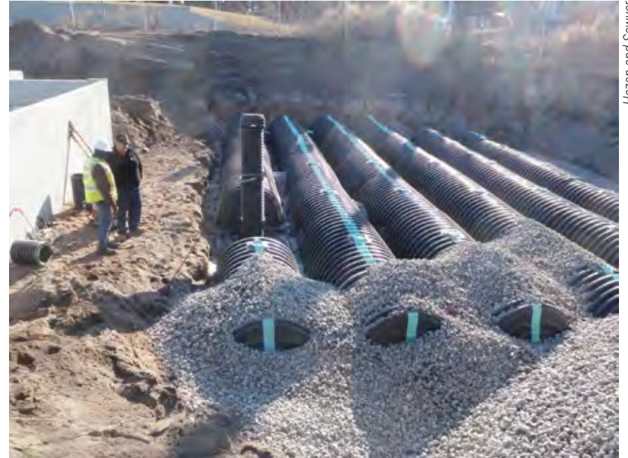
Perforated pipes in New York, NY.
