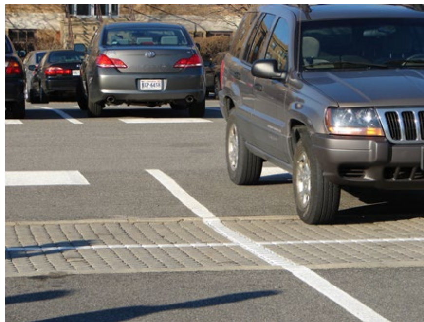
Permeable pavers installed at the downgradient end of parking bays collect surface runoff and allow it to infiltrate.
