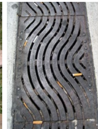
Figure 4-28. The small spaces in this grate are clogged with cigarette butts, which block drainage and are difficult to remove.
