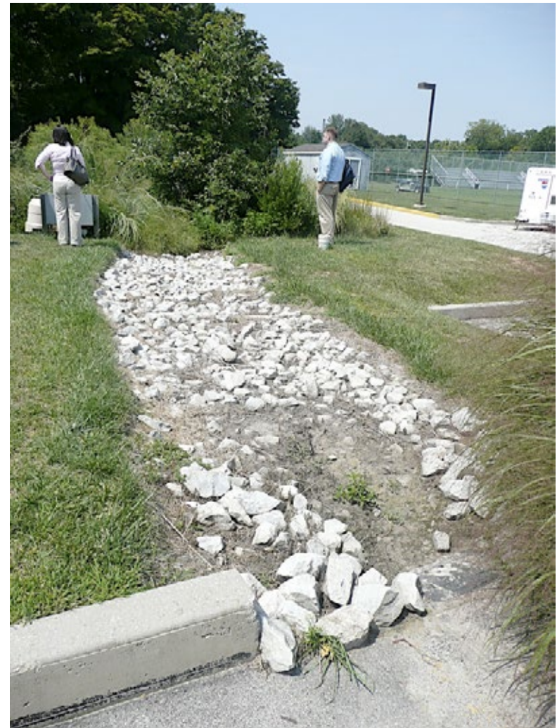
A sediment forebay provides pretreatment for parking lot runoff entering a bioretention cell at Villanova University, PA.
