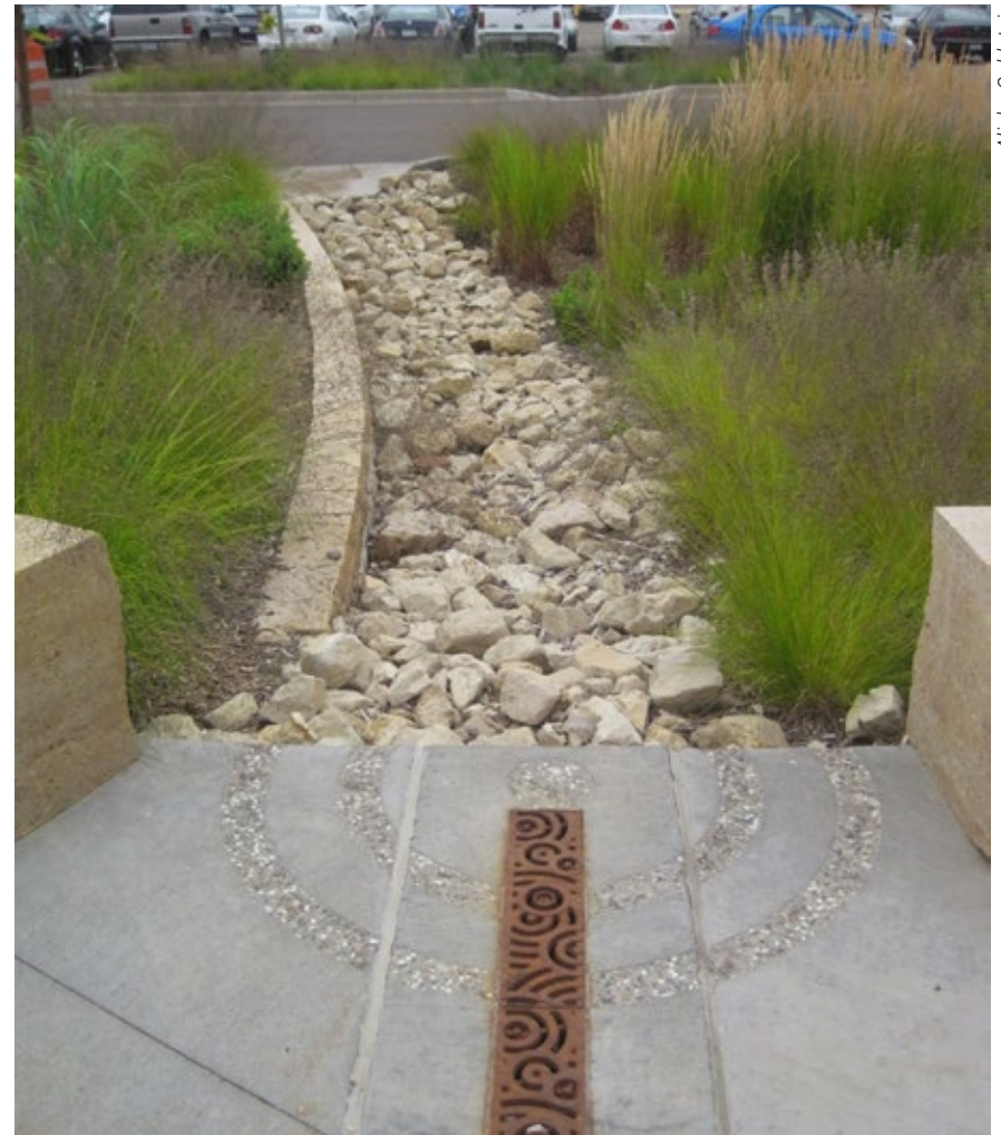
A sediment forebay provides pretreatment for a rain garden in Maplewood, MN.
