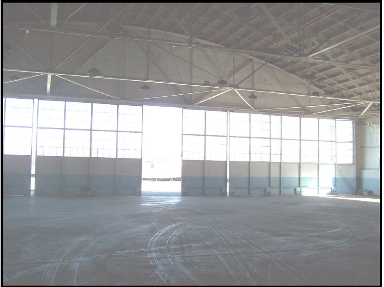
Figure 36: Open interior of Building 180, showing the interior side of the hangar doors and steel arched roof trusses.
