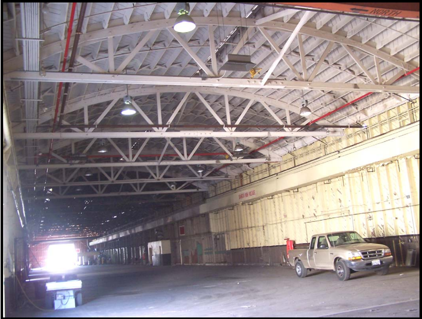
Figure 17: The interior of Building 121 showing the wooden roof trusses and stud wall construction. This view is from the west end, looking east.
