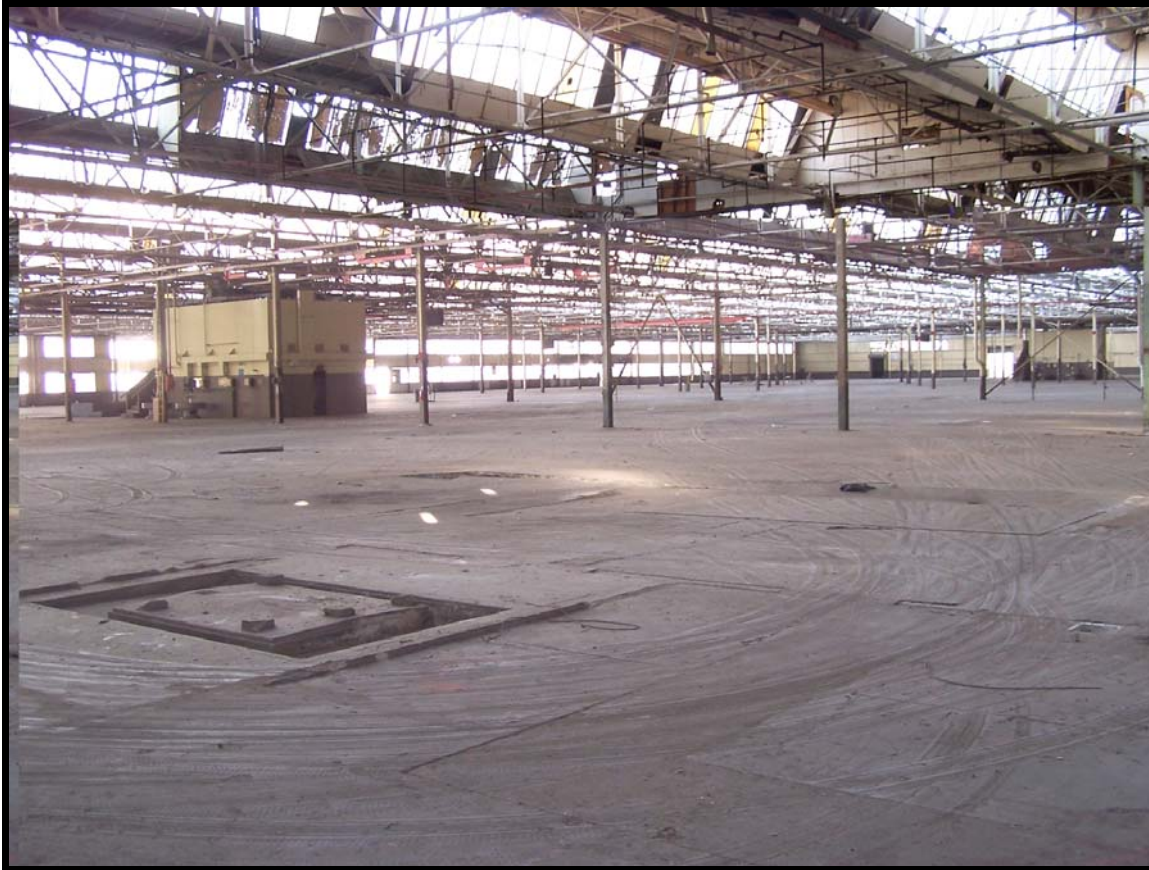
Figure 14: The large open interior of Building 120 illustrating the amount of light provided by the combination of monitor windows in the saw tooth profile roof and rows of continuous rows of windows along the building's sides.
