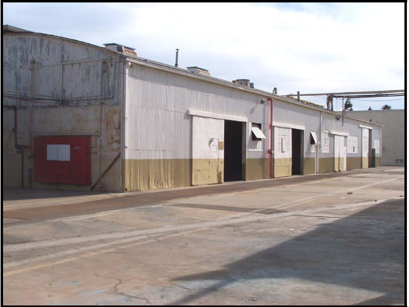
Figure 28: The northwest corner of Building 160, showing the west façade. Note the pairs of hanging doors.
