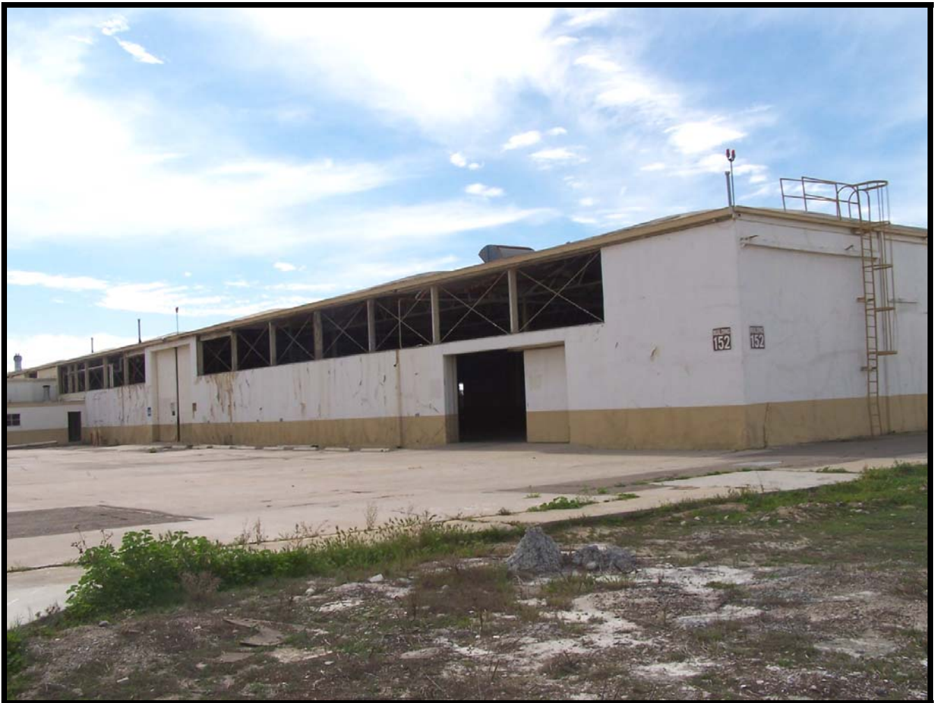
Figure 24: The northeast corner of Building 152, showing the east façade. The rows of steel framed windows have been removed.
