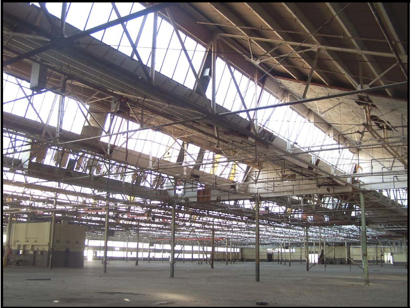
Figure 15: A close up view of the steel framing and monitor windows of the saw tooth profile roof in Building 120.
