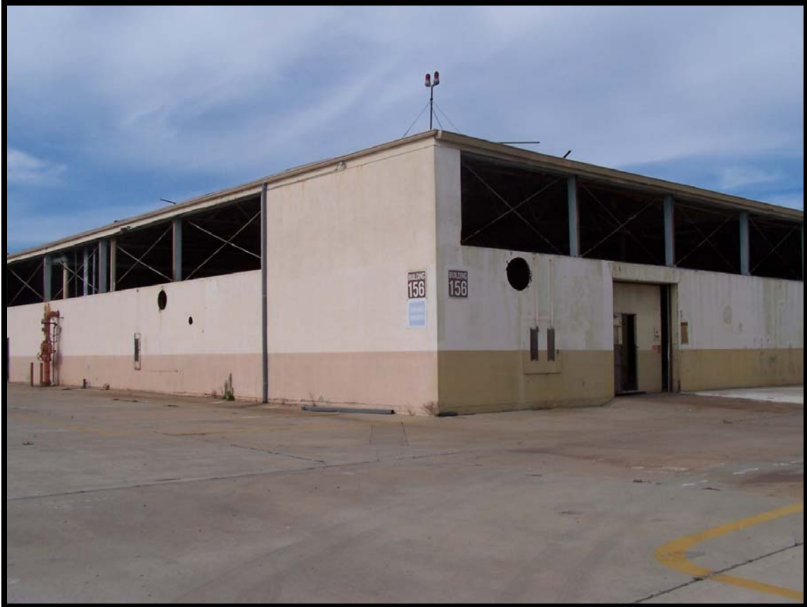
Figure 26: The southwest corner of Building 156. The rows of steel framed windows have been removed.
