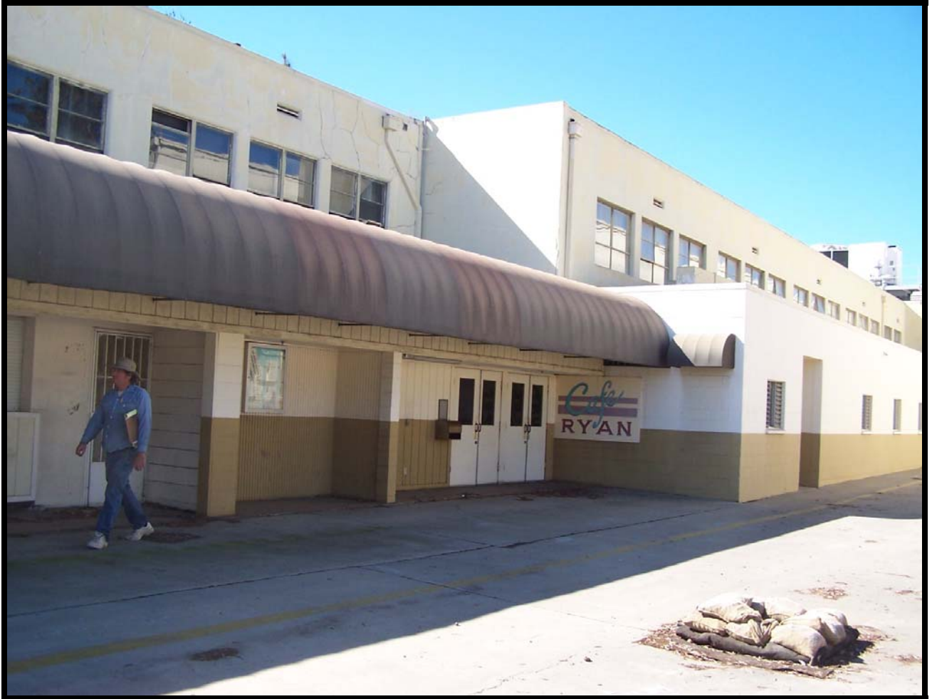
Figure 6: The back (north) side of Building 102, showing the variety of window and doorway placements.
