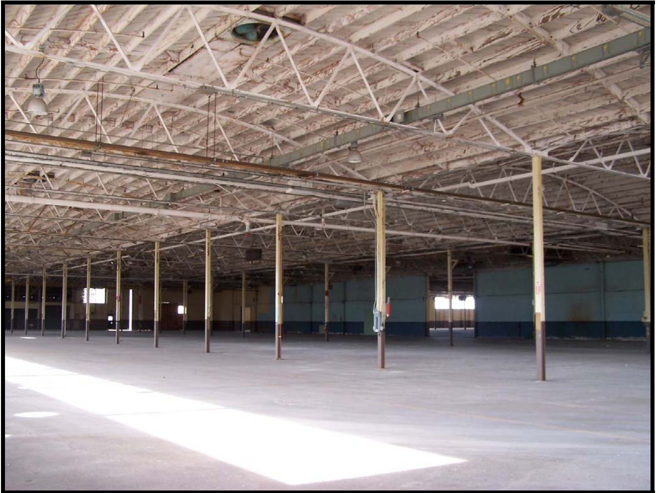
Figure 27: The large open interior of Building 156 showing the arched steel roof trusses supported by steel "I" beam posts. The opening near the far center of the photo leads to Building 152.
