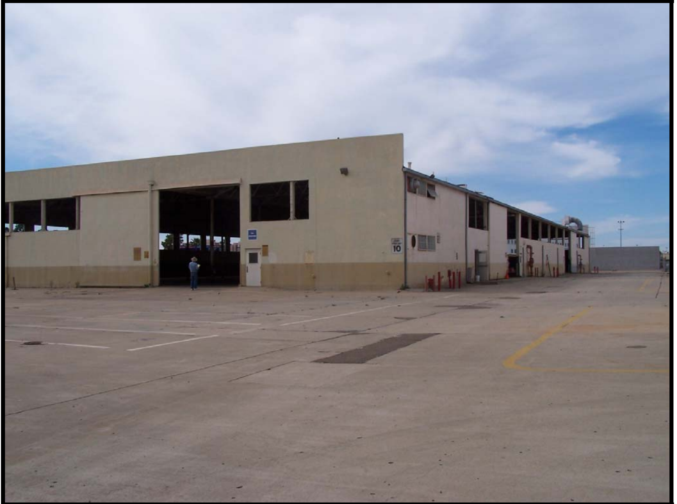
Figure 18: The northeast corner of building 131. Note the large hanging door on the east façade. The rows of steel framed windows have been removed.
