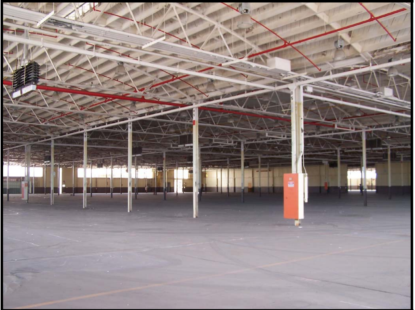
Figure 25: The large open interior of Building 152. Note the steel arched roof trusses supported by "I" beam posts.
