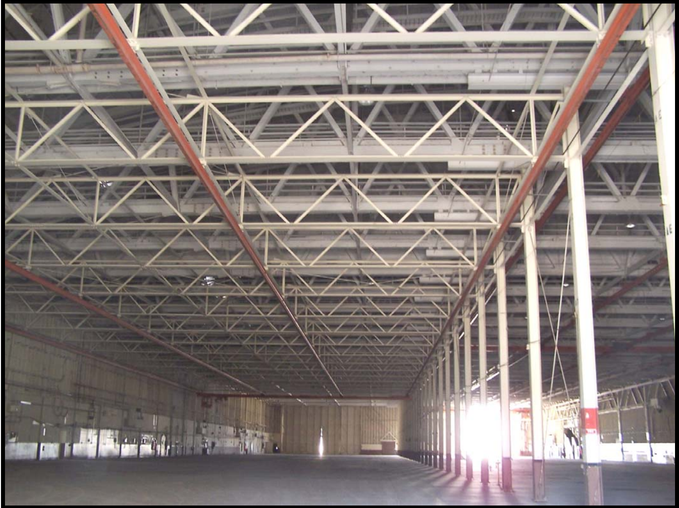
Figure 20: The large open interior of Building 140 from the east end looking west.
