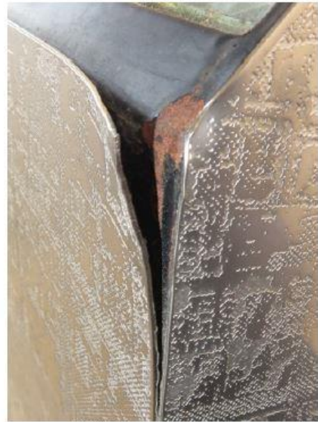
Detail of corroding framework.
