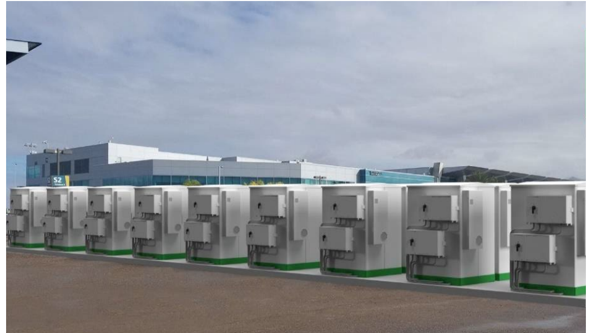
Battery Storage Units
