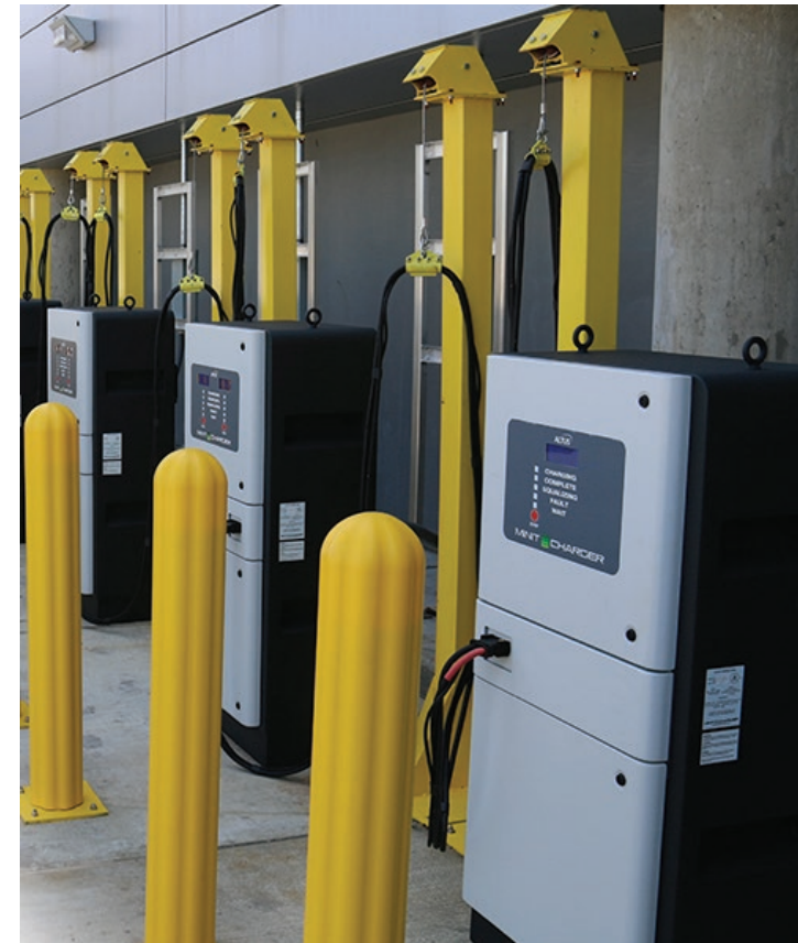
Dual-port EV Chargers
