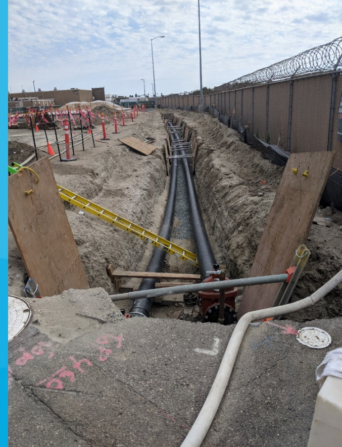
Underground Fuel Pump Lines
