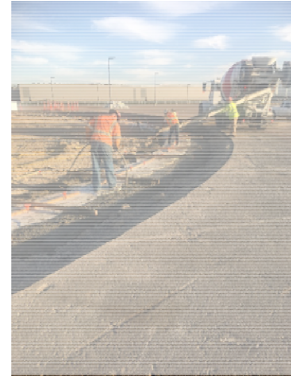
3000 psi concrete being poured around the foam templates to form guide wall which will contain the secant pile system
