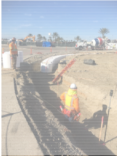
Excavation of 8' wide x 4' deep trench around perimeter of proposed tank in area of guide wall for pile system
