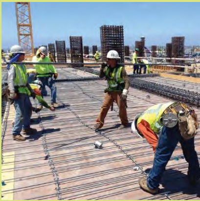
Approximately 6,000 workers are employed in the construction of the Rental Car Center.
