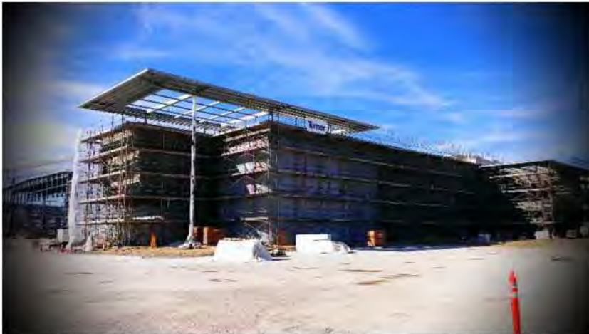
Construction is under way on a new complex serving general aviation aircraft.
