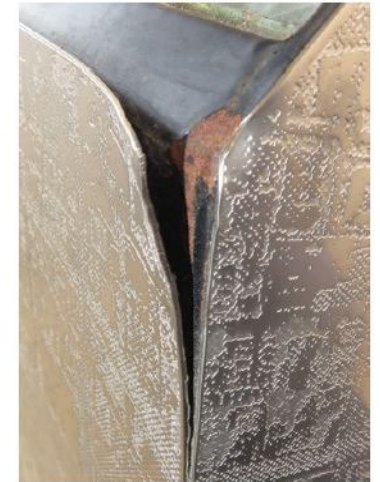
Detail of corroding framework.
