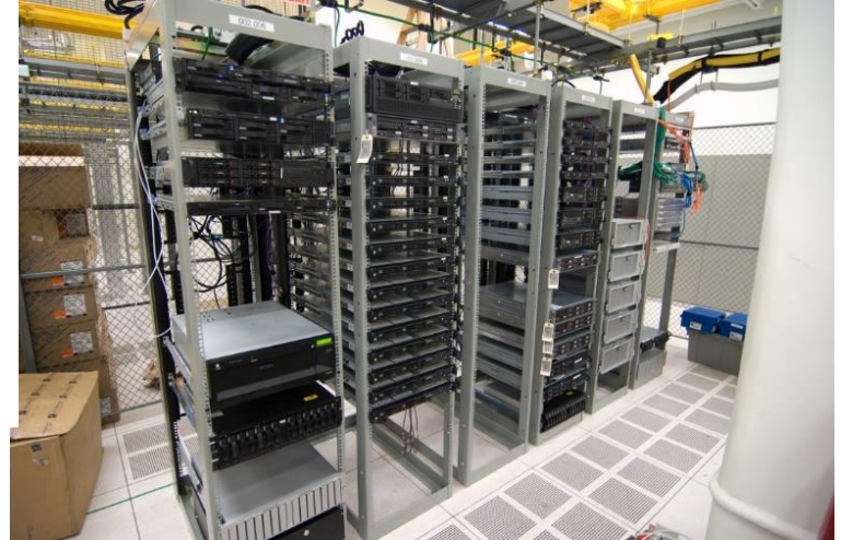
Examples of Server & Storage Hardware/System
