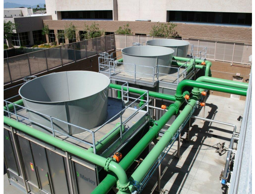
Example of Cooling Tower
