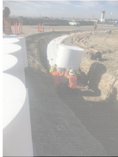
Foam templates being installed into trench using rebar to mark drilling location for secant piles
