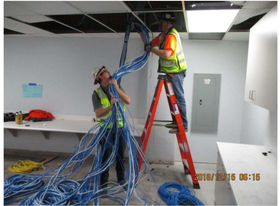
T2E- New Alaska Operations Room
