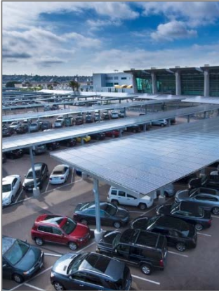
Onsite Renewable Electricity & Batteries [Strategic Energy Plan]
